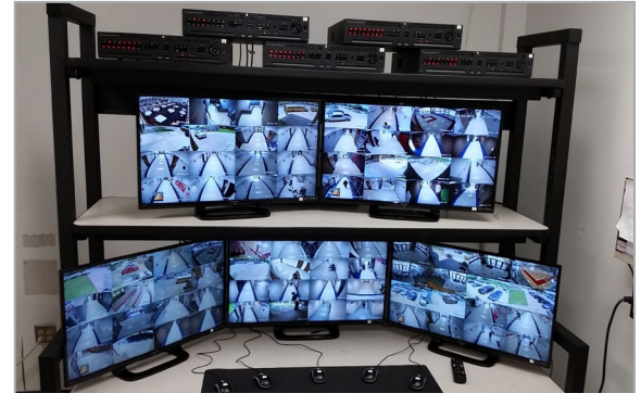
The new security cameras are installed and running at Sam Houston High School, the first AISD high school to receive the new cameras.
